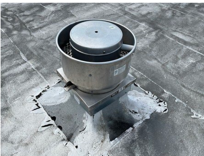
23 - TYPICAL EXHAUST FAN
