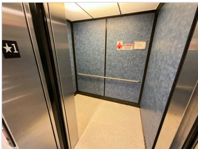
LOBBY LOOKING AT CABS (WITH DOORS OPEN)
