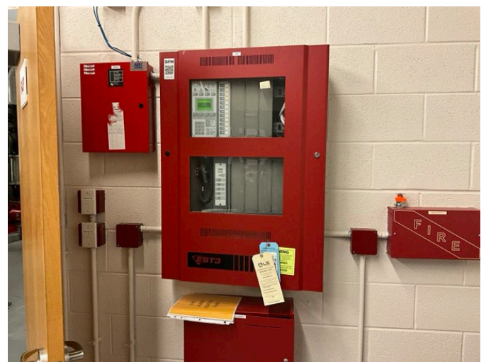
18 - FIRE ALARM PANEL
